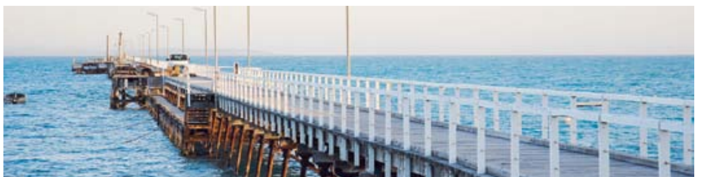
Work on upgrading Beachport's jetty is due to begin mid this year.
