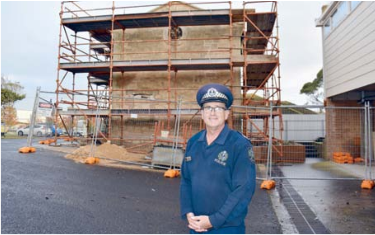
Facelift for lock-up: Pleased to see progress on the historic former lock-up is Senior Sergeant officer in charge of the Millicent police station Rick Errington.
