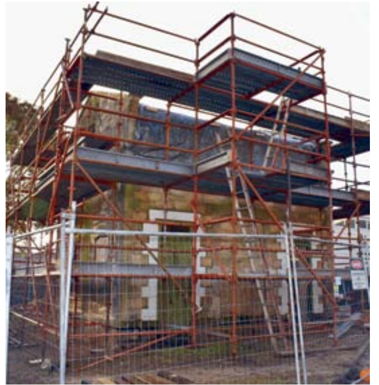
Restoration continues: The historic site is undercover in black plastic and scaffolding waiting for next year's planned reveal.
