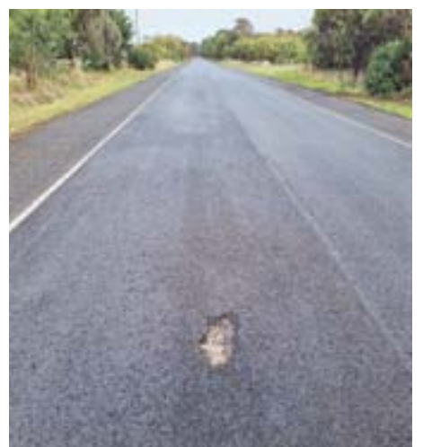
This hole appeared on the road to Rendelsham within days of roadworks being completed there. The hole has since been repaired. Picture: SUPPLIED
