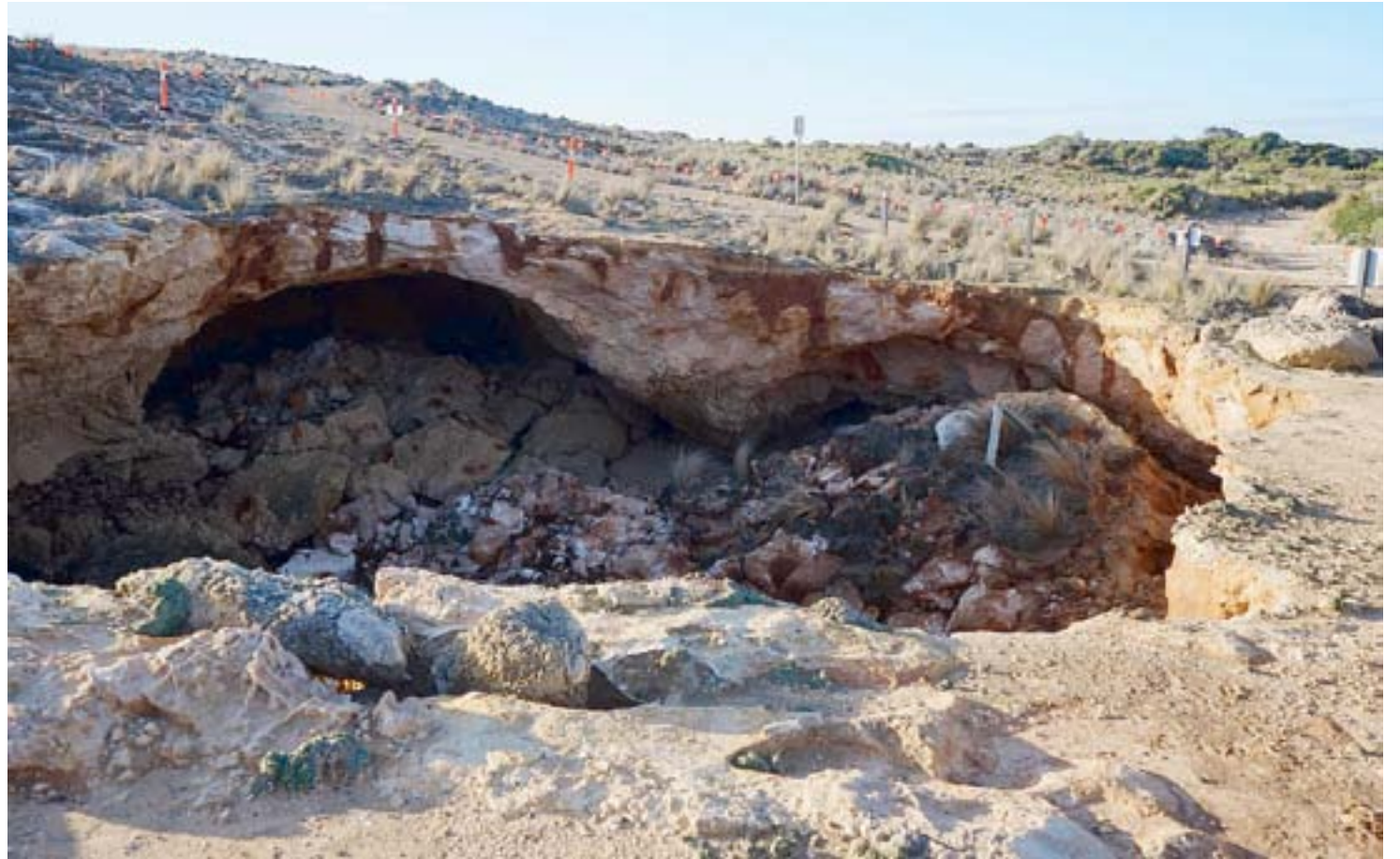
Hole in the earth: The damage to the Woe Hole has caused a significant opening to the surface.
