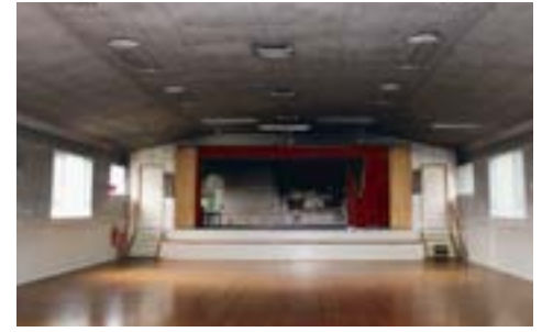
The main church hall has suffered smoke damage to the ceiling and walls.
