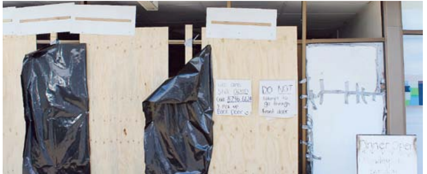
The front of Lien 88 takeaway in Davenport Street has suffered significant damage from the crash.
