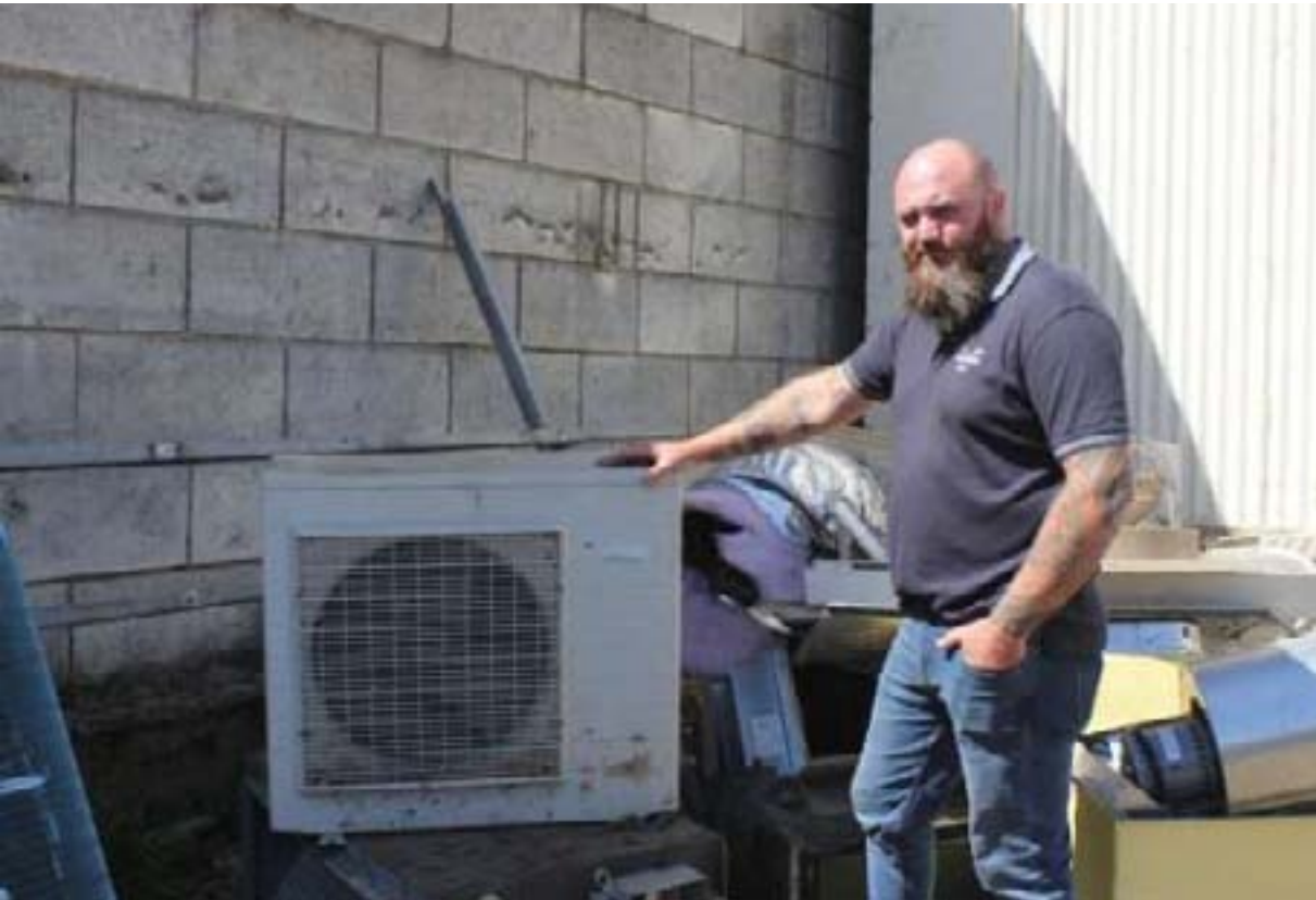
Kieran Swift with a similar unit to the one dragged over 40 metres to the rear of the premises.
