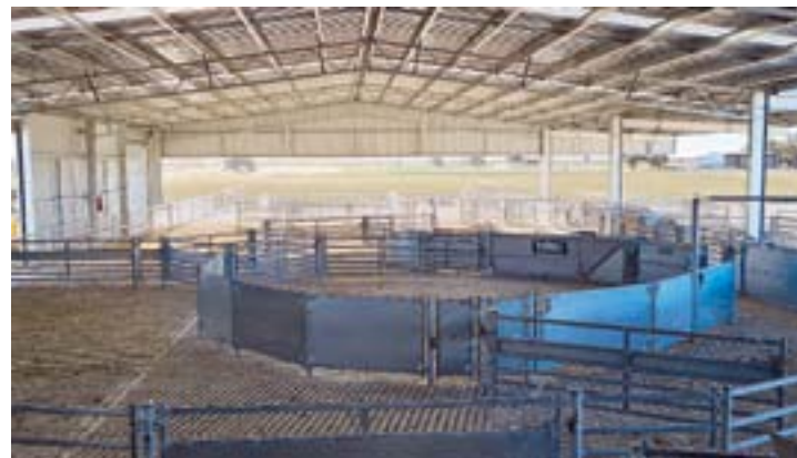
Yard Cover: A 58.5m x 18m x 4.2m ram sale shed and yard cover built by Action at Brimbago SA. View more shed builds at actionsteel.com.au .
