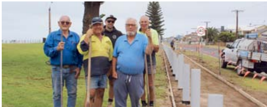
Lion's members Wayne Green, Ash Dearman, Ben Clark, Hayden Mansell and Mike Coonan prepare the path for the concrete pour.
