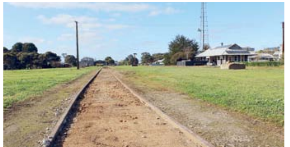
Excavation of the rail line is underway to prepare it for bitumising.
