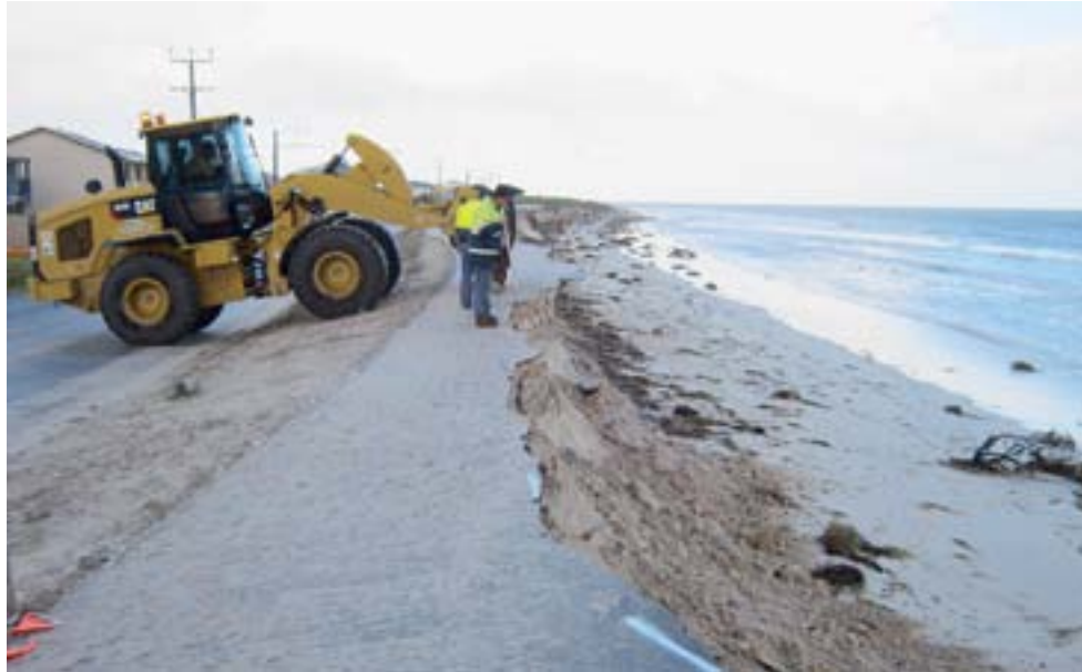
PLAN IN PLACE: Kingston District Council chief executive Nat Traeger said the new $2.6m seawall extension would hopefully prevent huge damage and cost for the Wyomi Beach sandbank.
