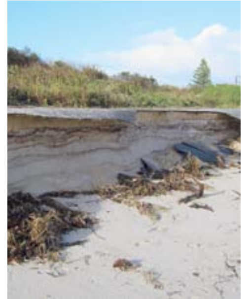
EXTENSIVE DAMAGE: Damage caused by erosion at Kingston's Wyomi Beach. Pictures: SUPPLIED
