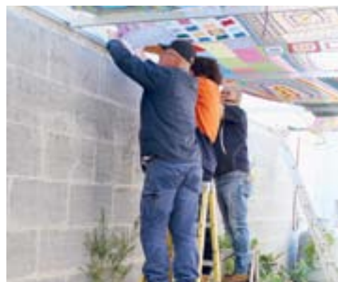
INSTALL DAY: Michael Pink, Fletcher Leopold and Dennis Muhovics secure the work to the frame.
